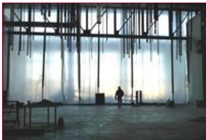
A construction worker walks through what will be the lobby to the grand ballroom in the new convention center.
